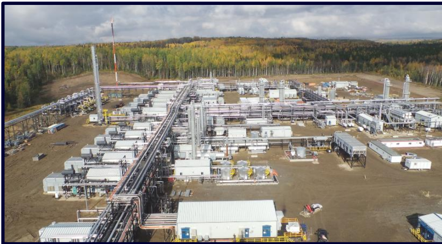
Glacier Gas Plant CCS Project installed
